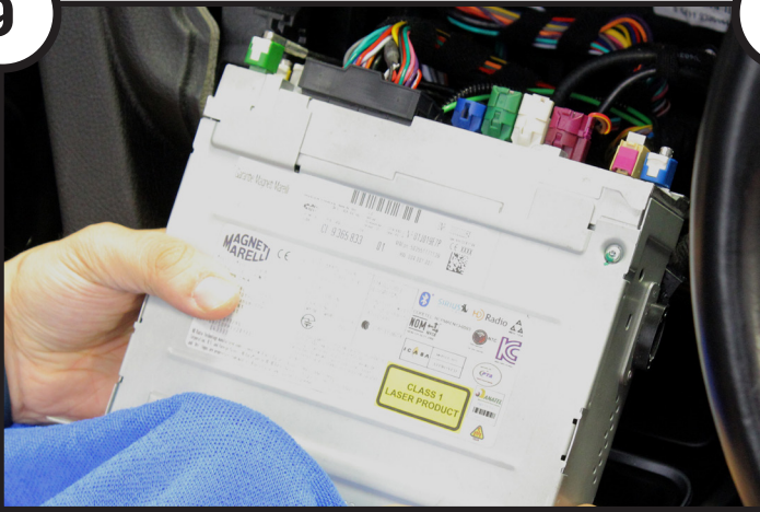
Remove the OEM head unit and disconnect all wiring to the unit. At this stage, the OEM head unit should be relocated into a suitable location at the rear of the vehicle.
